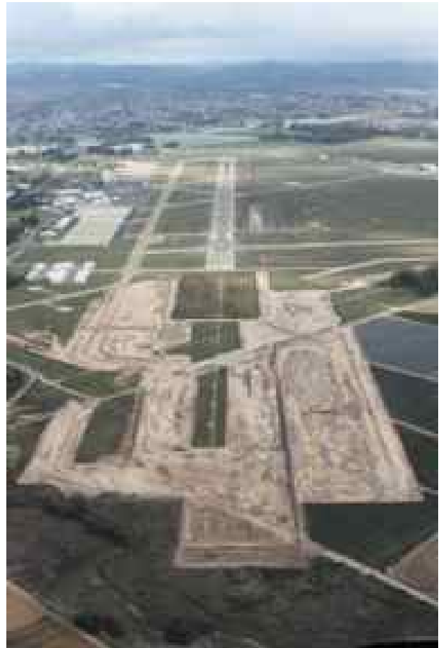
Aerial view of Phase one of the Runway Extension Project. Phase Two is due for completion by the end of 2011.
